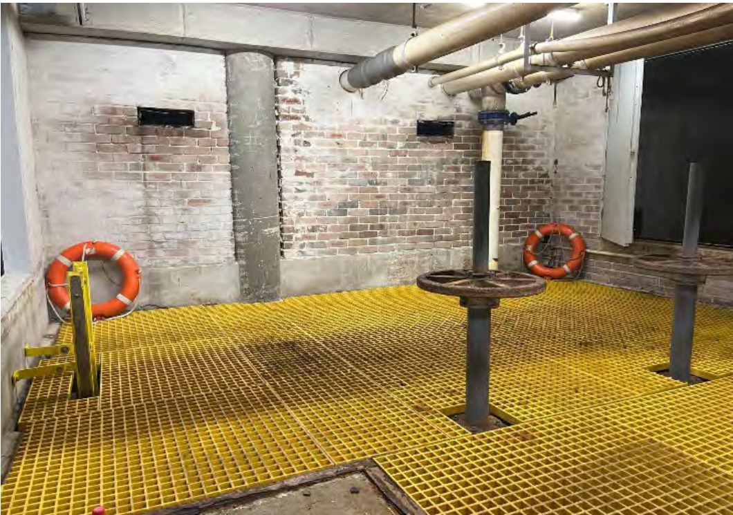
Figure 19 Seawater pit and valves in the basement
